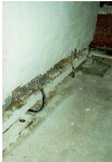
Figure 14. View of bottom plate after test (Photograph P. Florence)
